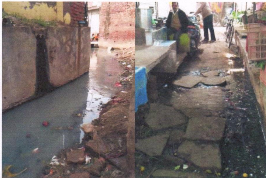
PHOTOGRAPH: DRAINS NEAR KATRE FATEH MAHMOOD KHAN AND SABZI MANDI
